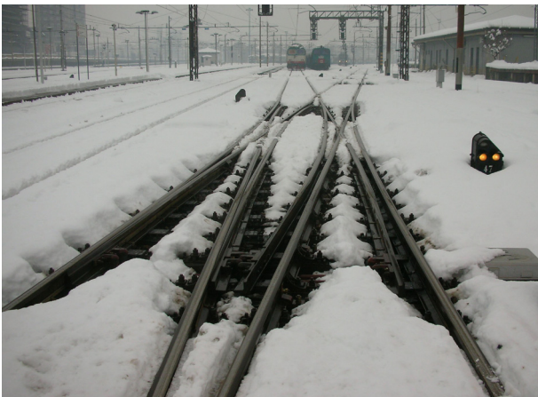
Typical Heated Points Systems - Milan, Italy.
